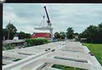
Precast Concrete Foundation Base Units are staged at / near the construction site in advance of construction.
