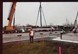
Precast Concrete Foundation Base Units are rapidly craned into position to provide the base for the building to be built on.
