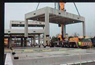
Precast Structural Building Units are rapidly craned onto and connected to the foundation bases to create the superstructure of the building.
